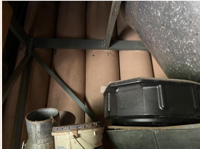
Dust collection filter bags (10 total) suspended from ductwork
