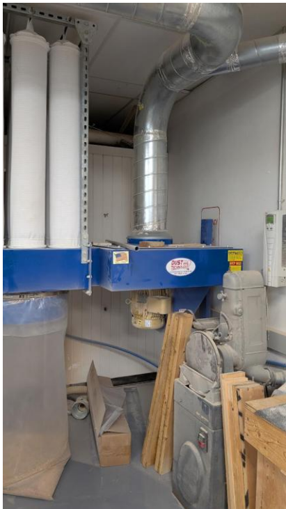
Dust collection system ductwork
