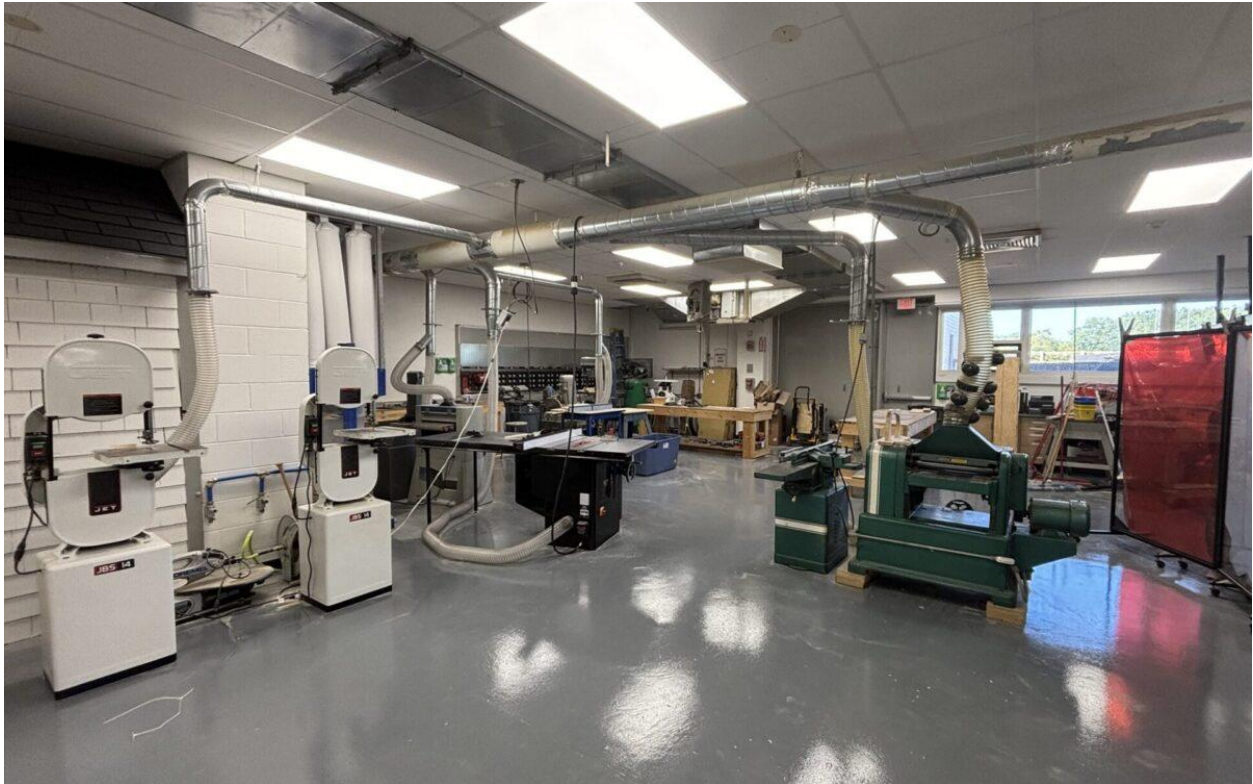
Ductwork and connections for the CHS Woodworking Shop dust collection system
