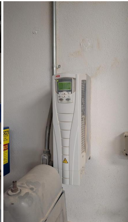
Dust collection system controller
